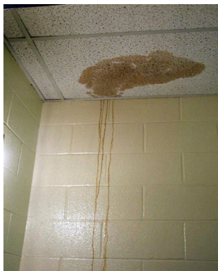
Roof leaks, like the one pictured left, can be found in every building in the school district
